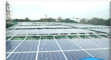
Indo-German Energy Programme – Green Energy Corridors and Energy System Optimization (IGEN - GEC) – Rooftop Solar PV Component
